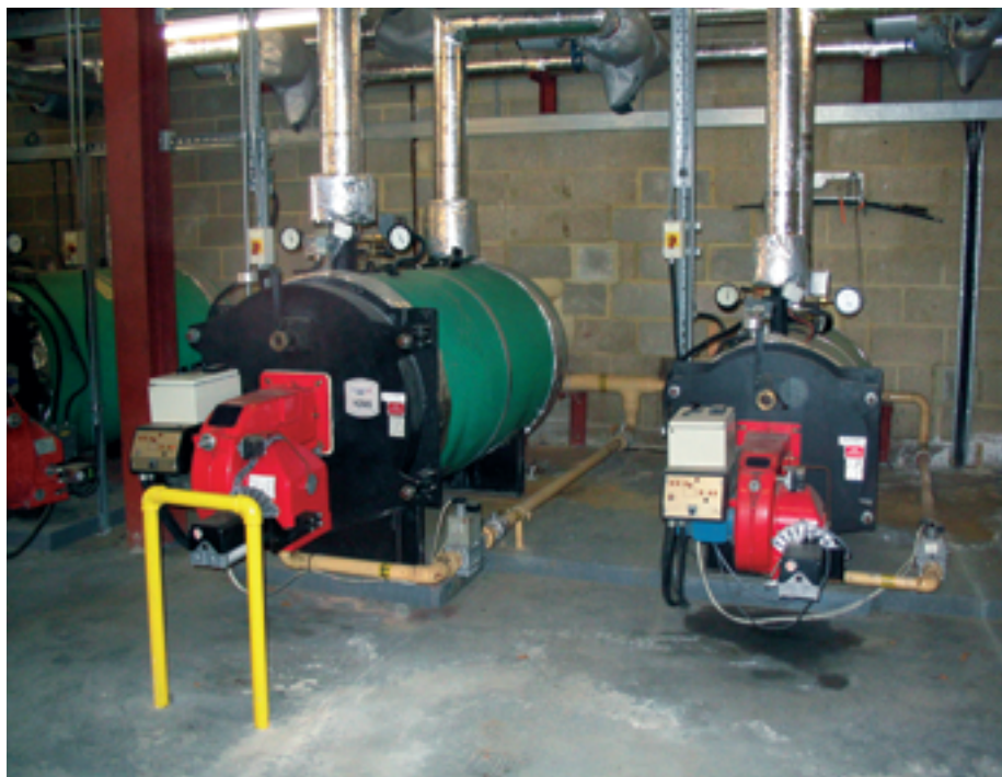
The updated fully modulating boiler system at Jealott's Hill
